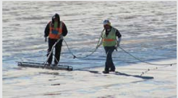
Figure 4. Water Puddle Testing
