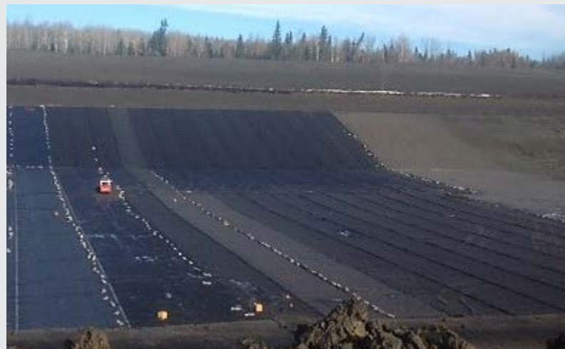
Figure 2. Geovolt® placement on the site
