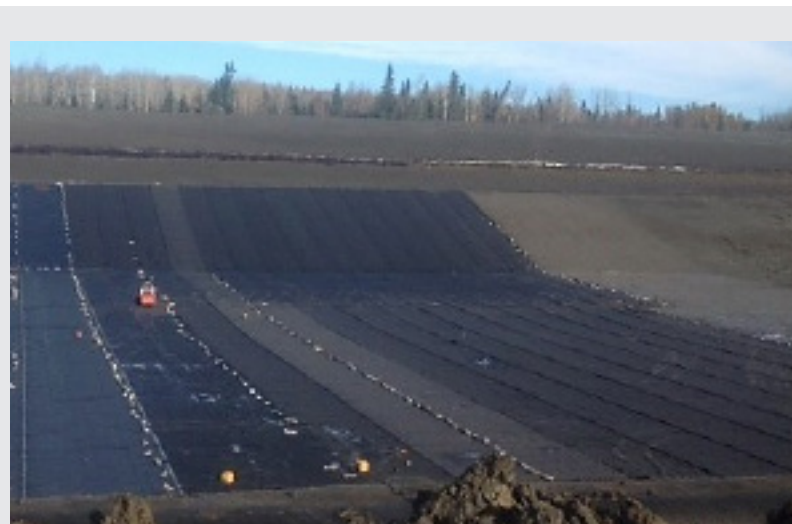
Figure 2. Geovolt® placement on the site
