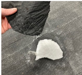
Figure 1: Damaged conductive layer.
