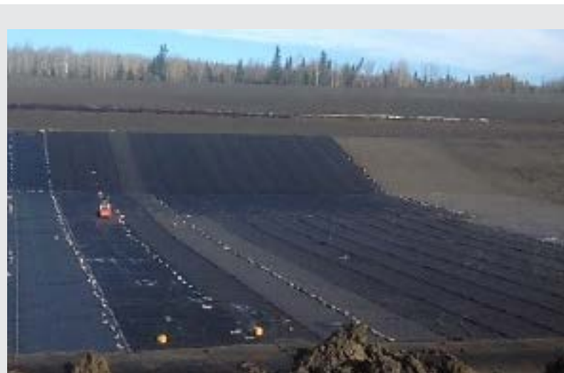
Figure 2. Geovolt® placement on the site
