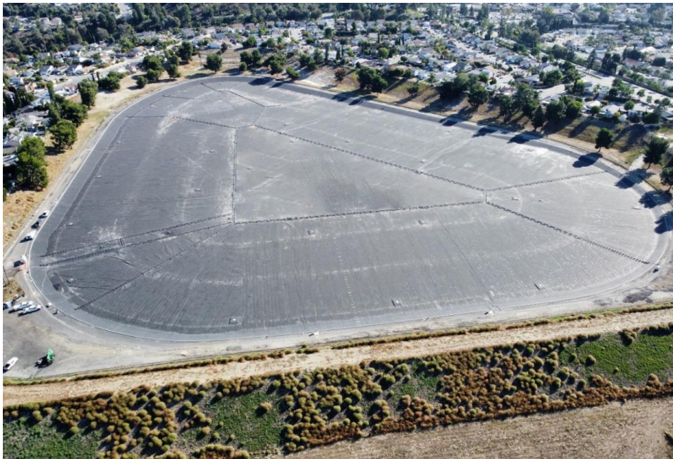
Figure 9. Aerial photo of completed CSPE Defined Sump geomembrane floating cover during water final filling and commissioning in 2023.
